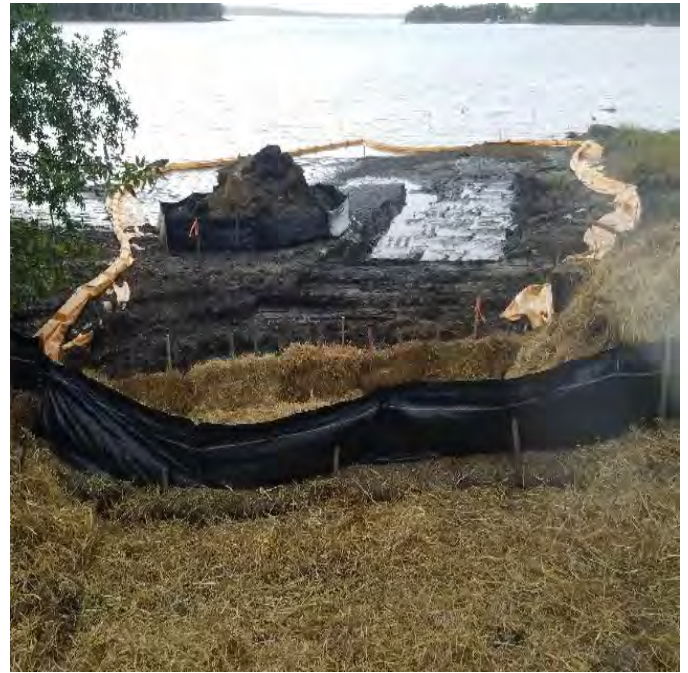
Fig 14: Blu Rock began excavating trench on the east side of the Bay. Viewing west. (10-7-19).
