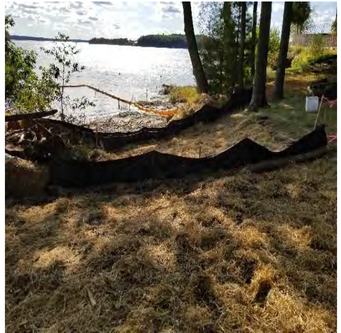
Fig 6: Sediment controls re-installed after test pits were dug on the east side of the bay near Beswick. Viewing west. (10-04-19).
