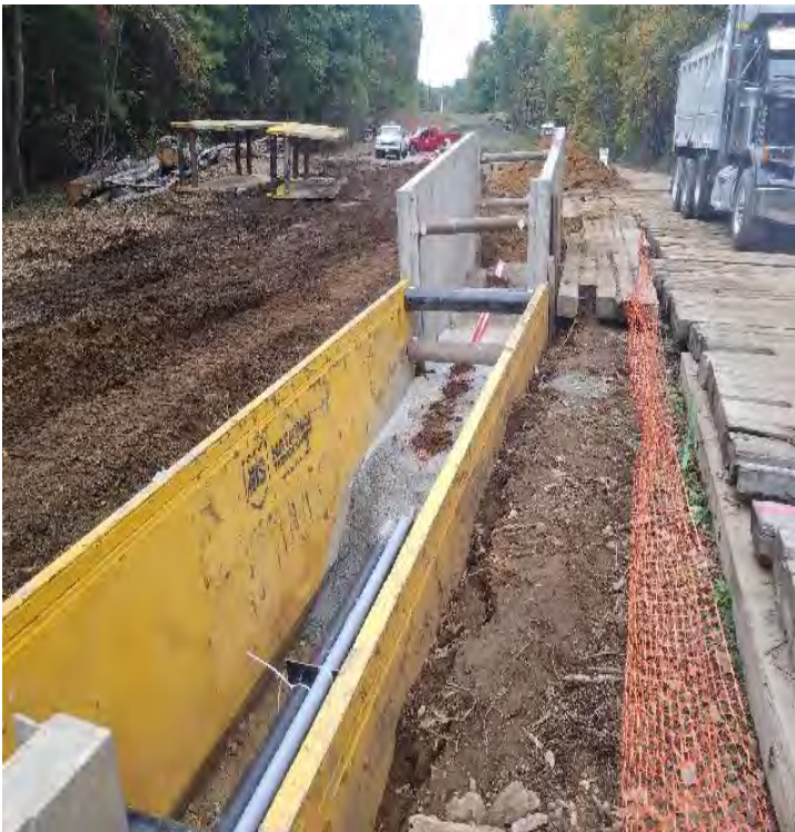
Fig 27: Duct bank at Str. 107. Viewing east. (10-9-19).
