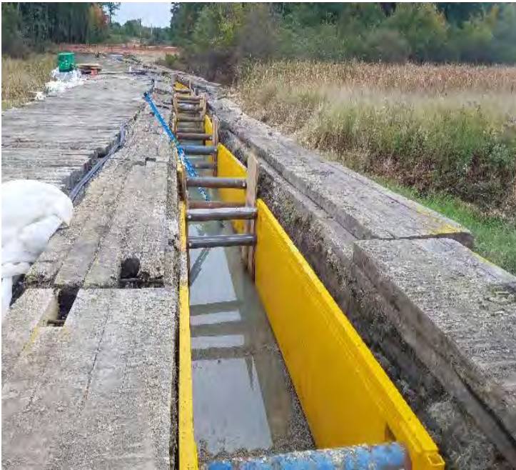
Fig 9: Overnight accumulation of groundwater in trench at Str. 106. Viewing west. (10-7-19).
