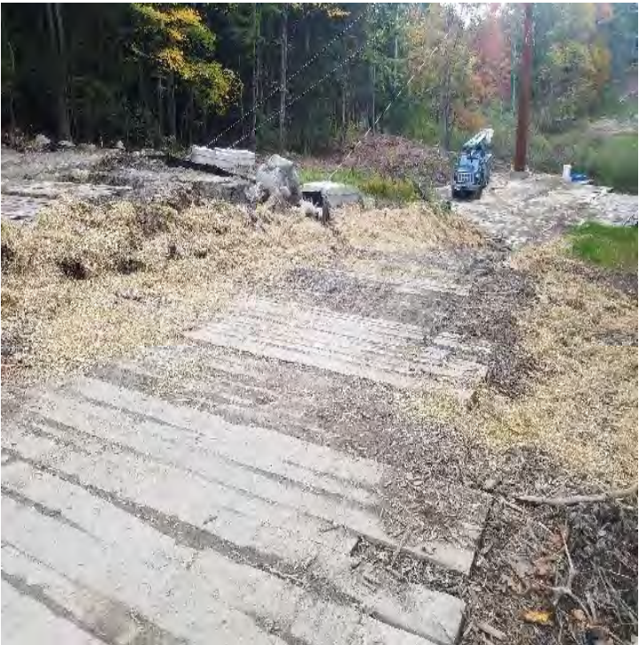
Fig 23: Exposed soils covered at Str. 29. Viewing north. (10-9-19).
