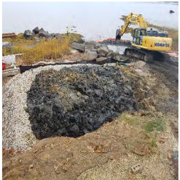
Fig 20: Blu Rock excavating trench on the west side of the Bay. Viewing east. (10-8-19).
