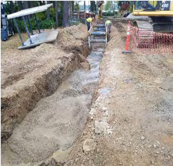
Fig 11: Duct bank at the Beswick property, Gundalow landing. Viewing west. (10-7-19).
